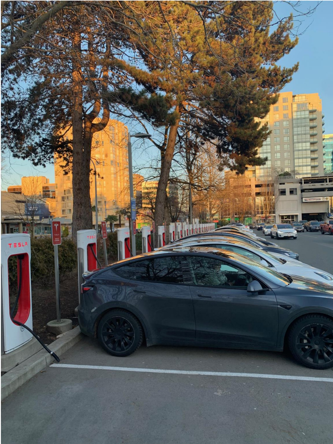
Electric Vehicle charging station in Richmond
